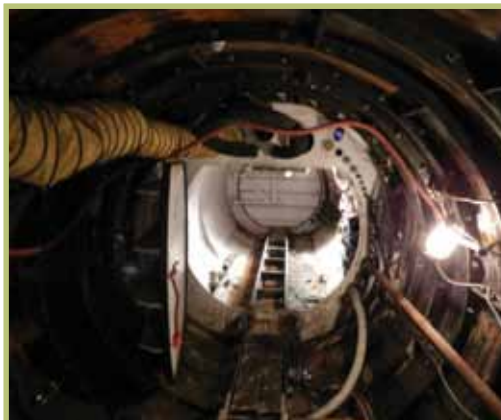
This photo was taken from inside of the tunnel. As you can see there is no latch on the door. The doors were held shut by the pressure of the air. The airlock was long enough to accommodate the spoil removal equipment.
